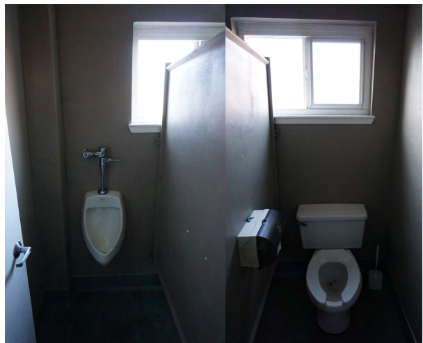
Firefighter's restroom: urinal and toilet
