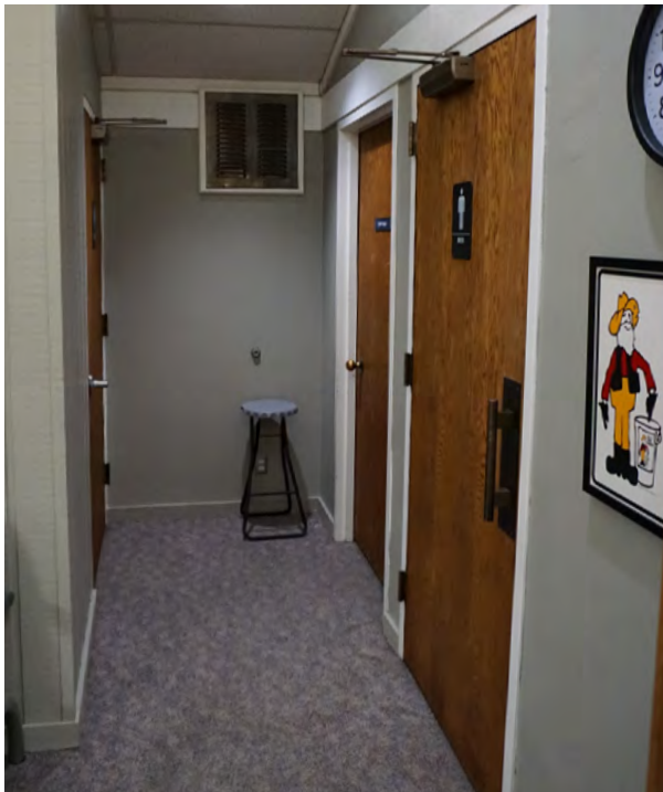
Public restroom access via blind corridor
