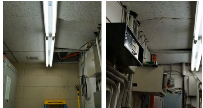
Damaged ceiling tiles with exposed wiring
